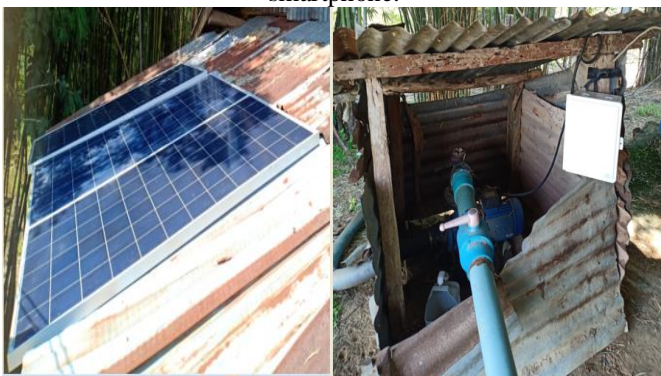
(c) Solar water pumping system
